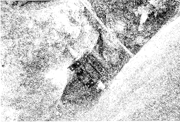
Fig. 3 - The TM71 instrument installed between the footwall and hanging wall and behind it the Bragg Gitter extensometer (the grey protective tube is visible).
