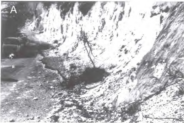
Fig. 5 – Surface faulting along the bedrock fault scarp near Senerchia: a) reactivated fault plane affecting striated, poorly cemented, eboulis , and displacement of the roadway; b) free-face at the base of the limestone fault plane. Photos taken on 04.04.1981, at close distance along the road behind the village; courtesy of Prof. Albert Pissart.
